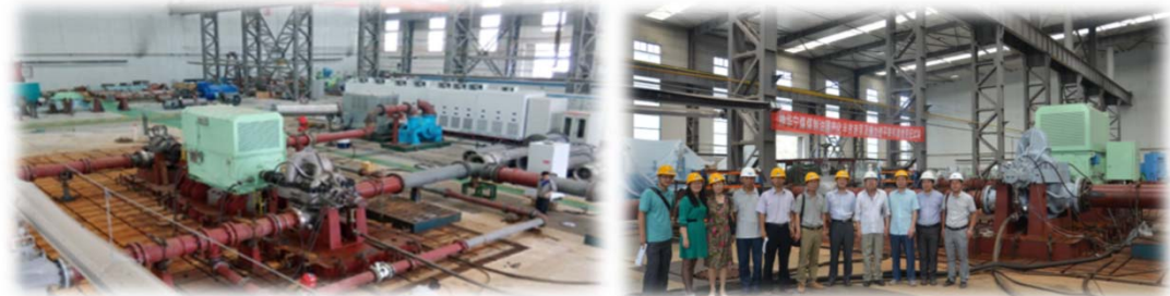
Joint acceptance of hot potassium alkali lean liquid pump for the world's largest Shenhua 4 million ton coal to oil project
